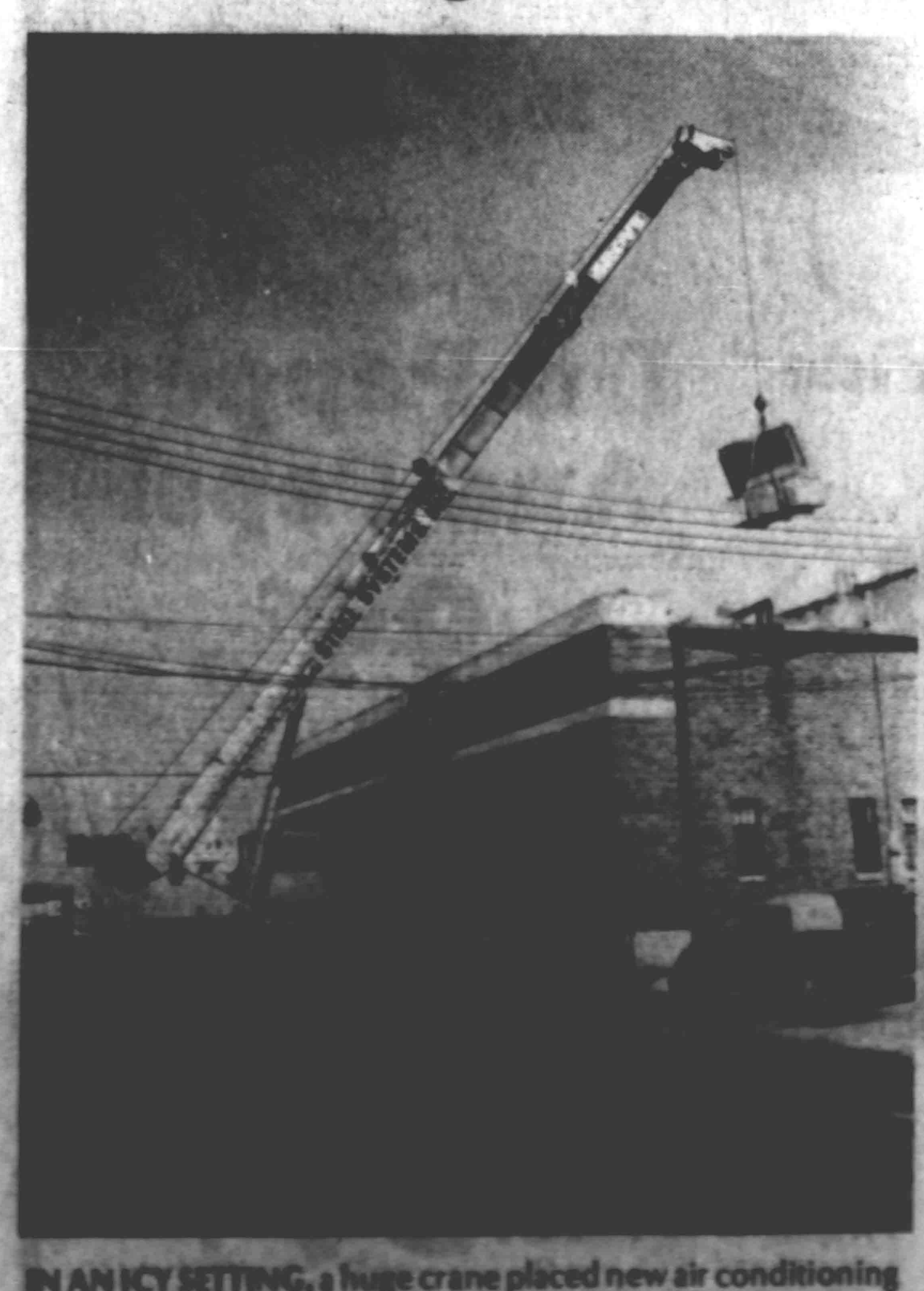
IN AN ICY SETTING, a huge crane placed new air conditioning equipment atop the Bank of Halls' main building Tuesday.
